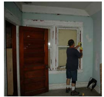
Assistant Keepers Building: Erik Maki chipping out window stops in order to remove the lower damaged window sash for restoration over the winter.
